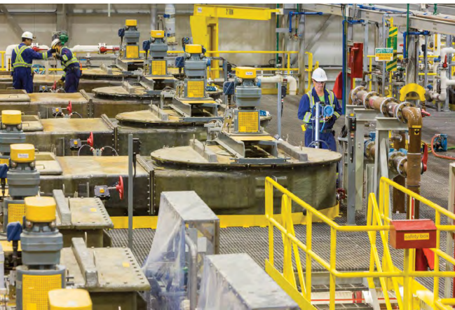
Uranium SX Plant, Canada (Photo courtesy Orano Canada)
